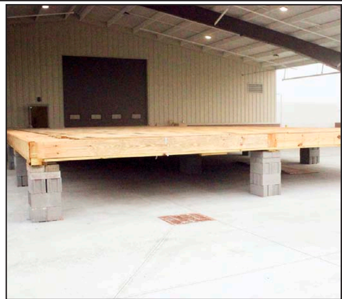
The CTAE Construction Pathway at Union County High is working on a Habitat for Humanity home build at the College and Career Academy, with the established flooring of a future home shown here.
